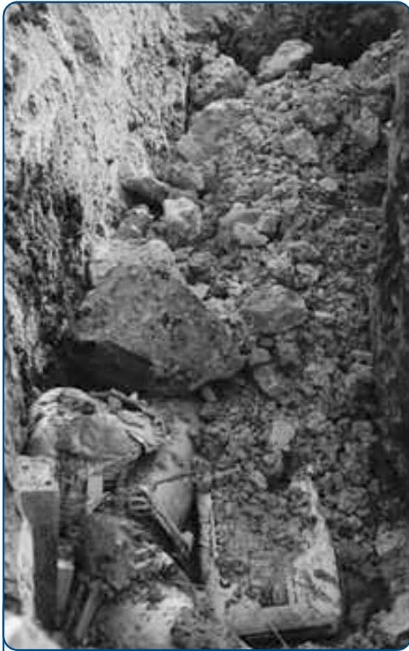
The backfill seen in this photo is of a much larger size than recommended. (Photo by Julie Black)
