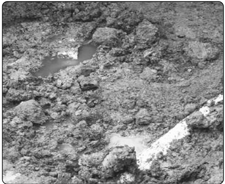
Wastewater rising to the surface or "ponding" as a result of a failed drainfield.
