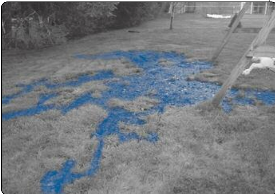
Damaged, waterlogged areas in the lawn over the drainfield indicate drainfield system failure.
