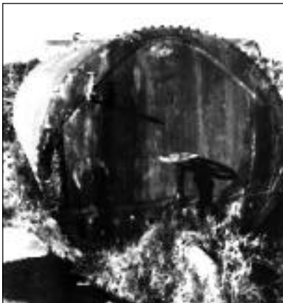
Every state needs help: This large rusty tank, found in California's Imperial Valley, is used as a pressure tank to pump water in a small Mexican-American community. The water is not treated for impurities or contaminants.
