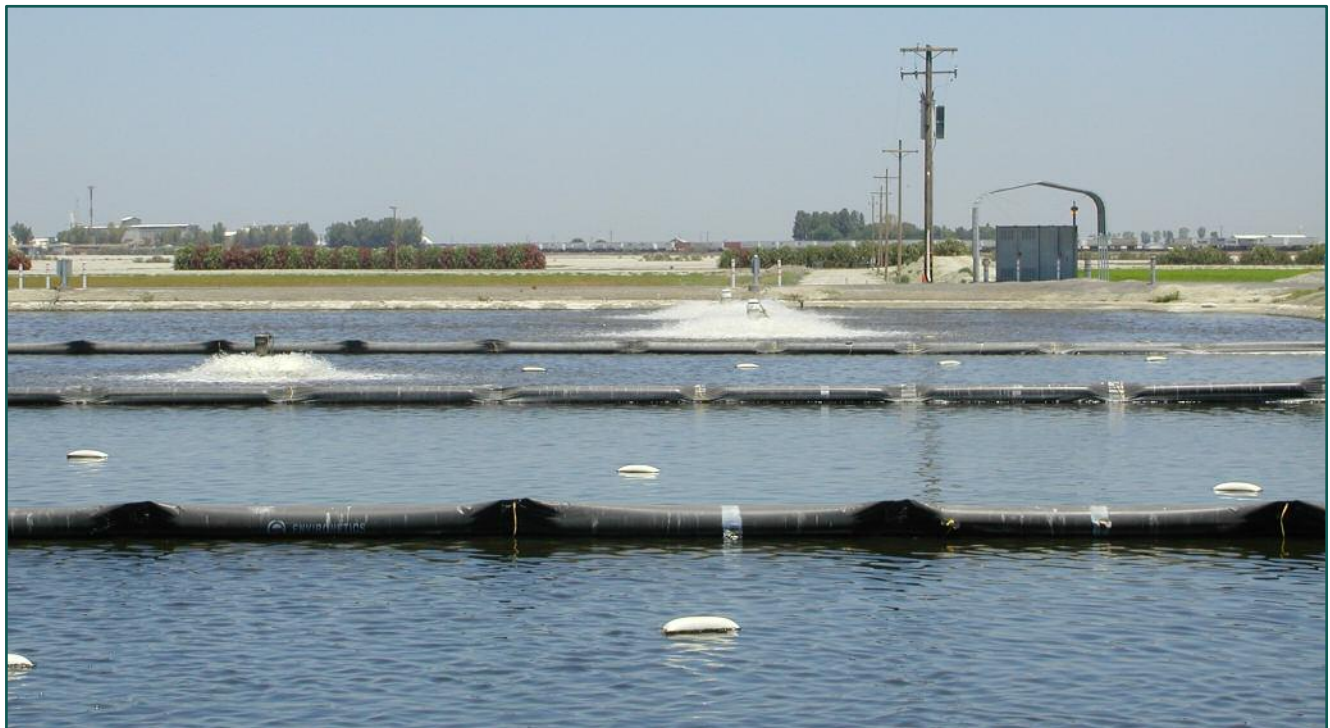
Photo 2 DPMC Aerated Lagoon Cells. The Motor Control Center With a New Sun Shed and Cell 1 Are Shown at the Top of the Photo. Floating Baffles Separate the Cells.
