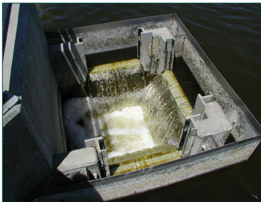
Photo 3 New Effluent Structure with Baffled, Adjustable Weir (Water-Level Control Planks Are Removed)
