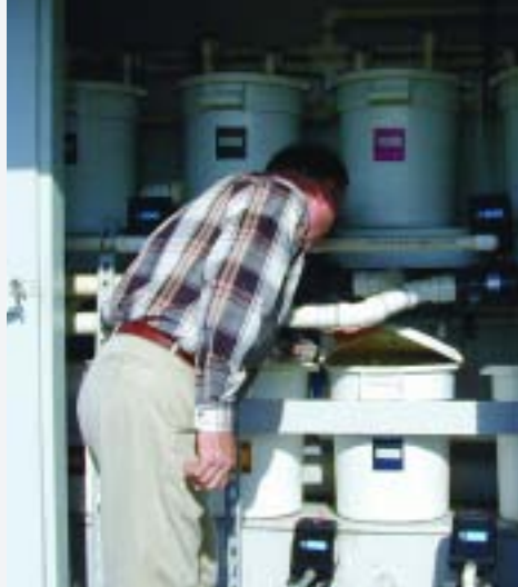
Checking the dosing containers.
