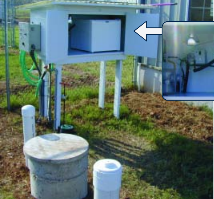
Sample collection enclosure with the refrigerator inside. The tee-cross and other risers associated with the system are in the foreground.
