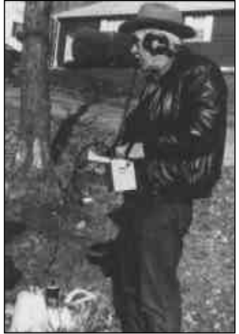
Testing for leaks at a small water district, Holt uses his detection equipment to check a fire hydrant. "Unaccounted for water loss" of 20 to 30 percent is common in small West Virginia water systems.
