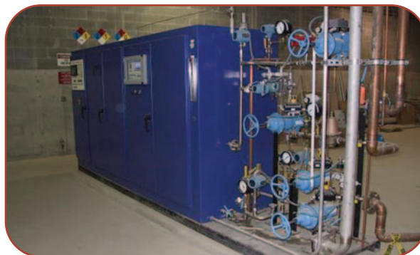
Photos Source: Wilsonville, Oregon Water Treatment Plant
